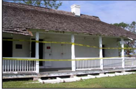
Snapped Rafter Tails
