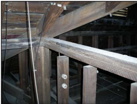
Roof structure dropping due to missing structural wall below
