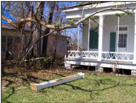
905 East Beach, toppled column
