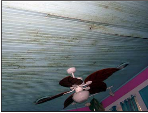
Mold and Water damage to Bead Board Ceiling
