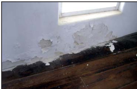
Inappropriate elastomeric paint trapping moisture in original bousillage walls
