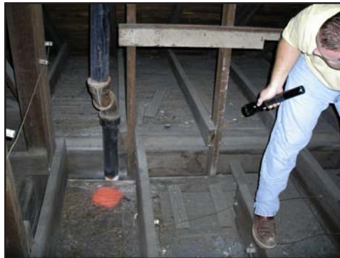
Plumbing stacks penetrating corner plates disconnecting ceiling joists
