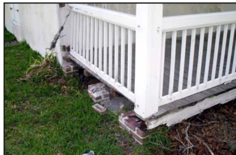
Termite damage typical to porch structure
