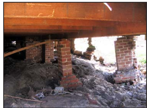
Damaged brick piers at Terrace Hill
