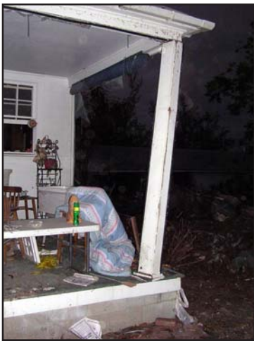
132 Davis, Porch Column Shifted
